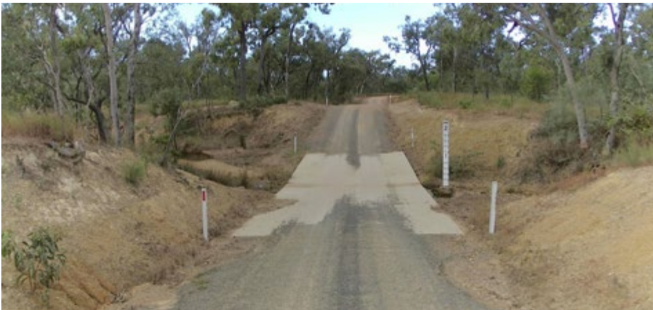
Figure 50: A concrete floodway installed at a creek crossing to reduce bed scour, but with associated erosion at the diversion track (Figure 54). Note downstream scour below concrete due to lack of rock protection; and rill erosion on batters.
