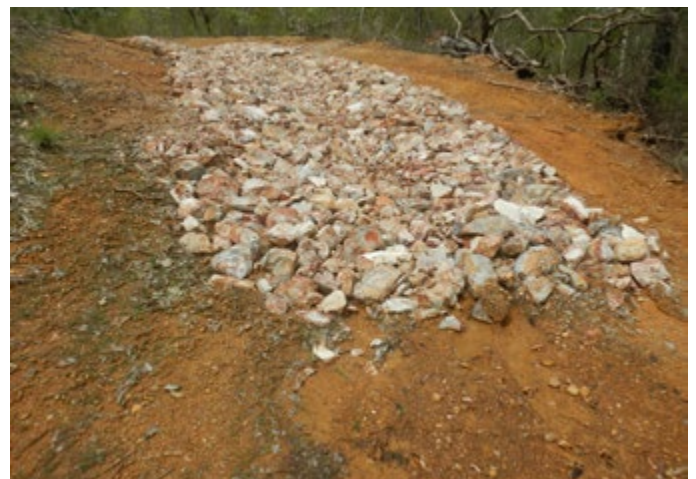
Figure 44: An incising V-drain outlet (top) and rock chute (bottom) at the same location to control erosion incision.
