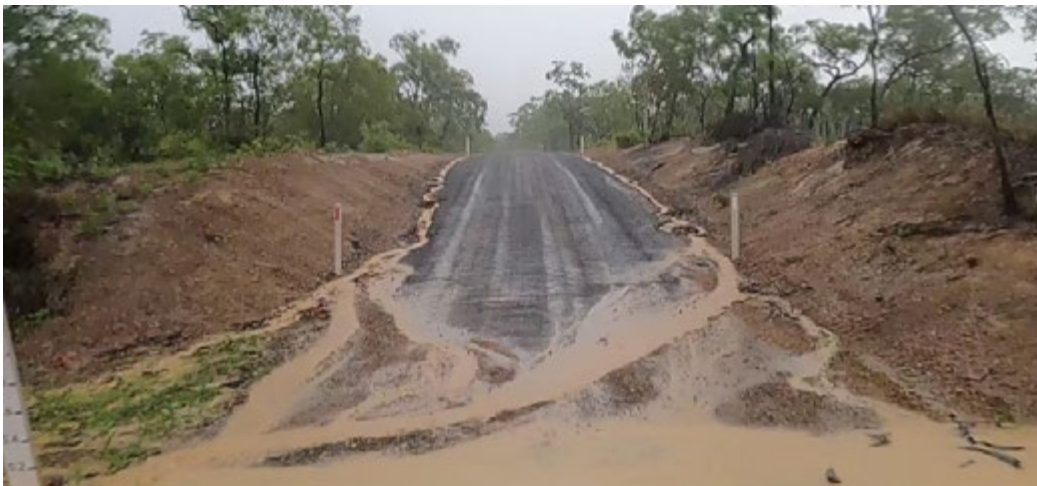
Figure 38: Table drains well connected to streams with few places to divert sediment laden water from bare batters.
